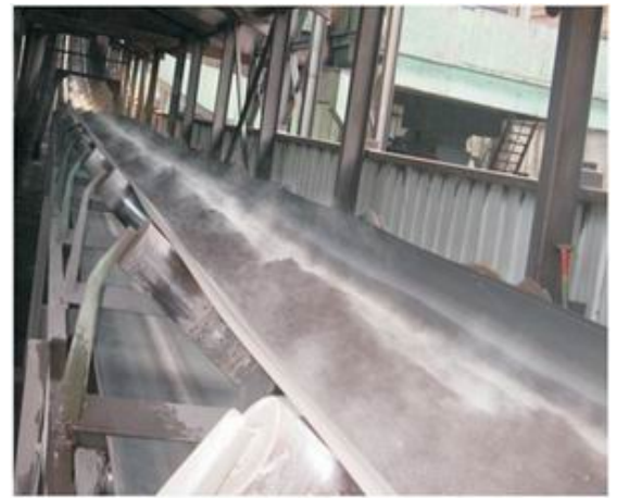
DT II belt conveyor
